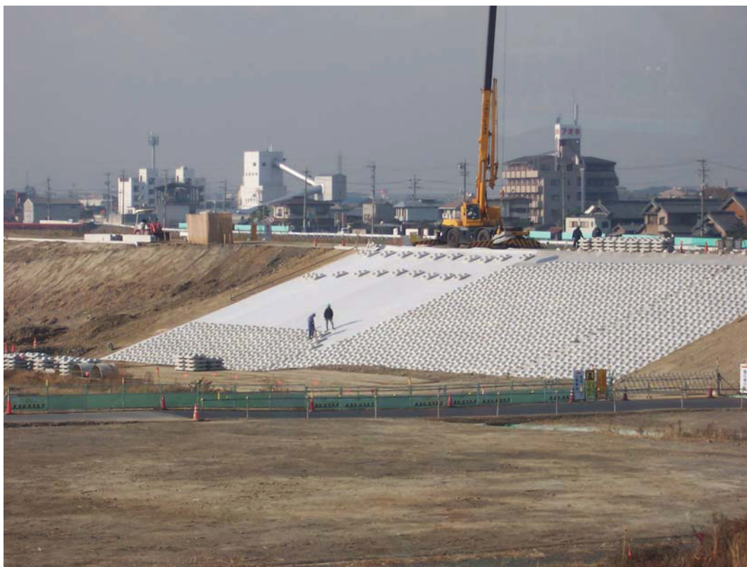
FIGURE 6-4: An example of an armored levee in Japan. SOURCE: Courtesy of Gerald E. Galloway.
